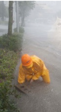
Bureau of City Appearance Action: draining sewage
